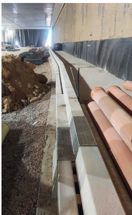
Tunel S52 Kraków AS-S200 K-T
